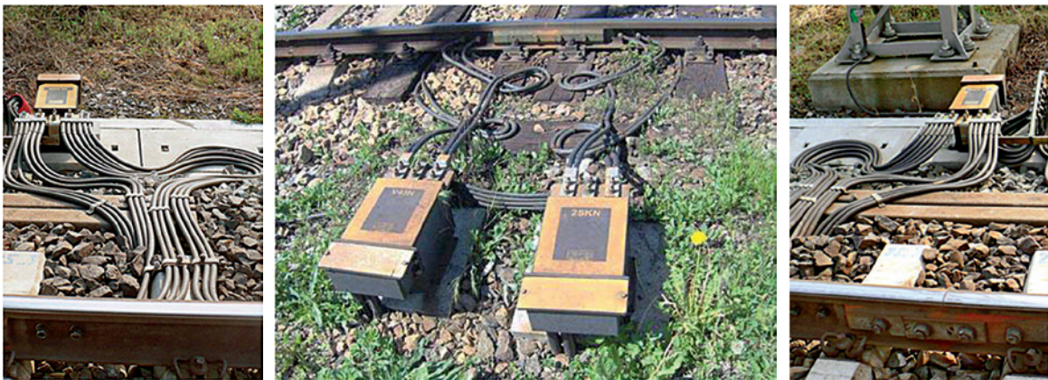
Picture: Track circuits (Photo: SŽDC)
