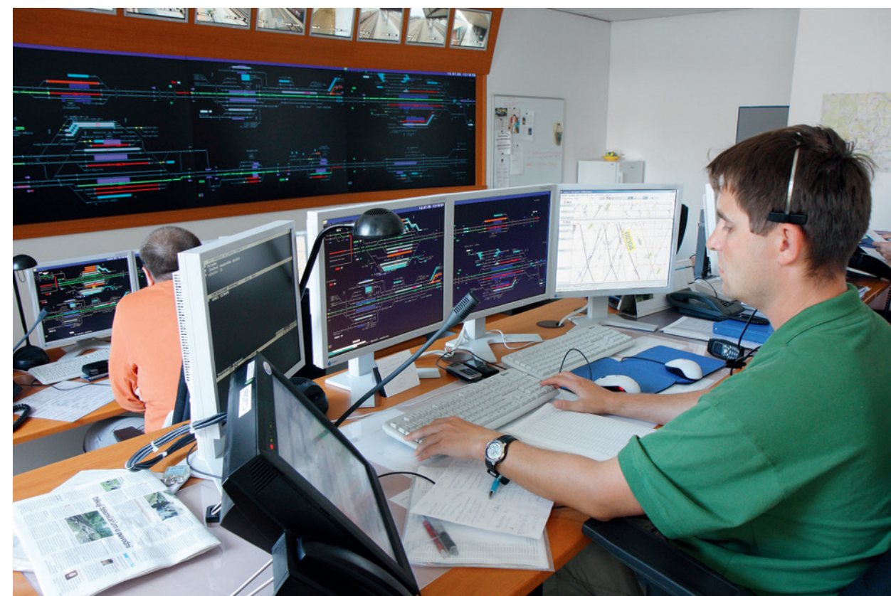
Picture: Work post of the Central Dispatch Station (CDP) Písek (Photo: SŽDC)
