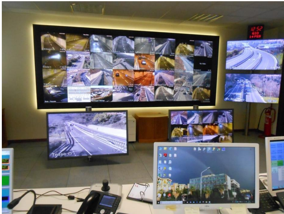
Figure 2.3: Traffic control centres: the backbone of digitalization for the infrastructure
