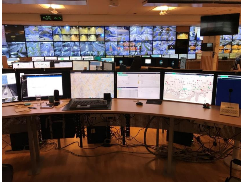
Figure 4.3: Traffic management centre in Finland (© Lone Dörge).
